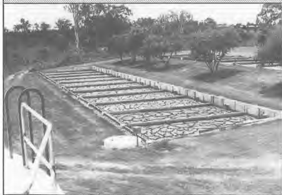
Sludge removal to drying beds (as shown above)
